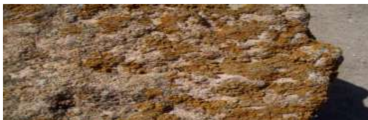
Fig. (15) biodeterioration of limestone
