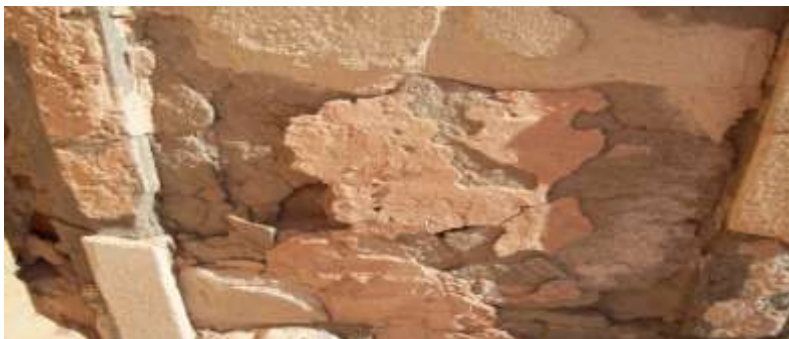
Fig. (17 ) deteriorated of plasters
