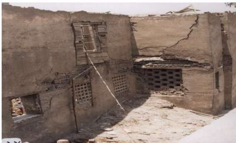
Figure (8). Present state of Wkallah Radwan Al-Fakari, before restoration processes.
