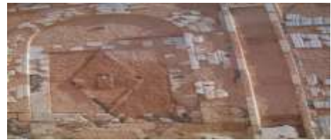
Fig. (12 ) Spallation of marble decoration slabs
