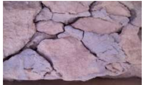
Fig. (10) Deterioration and disintegration of unsuitable mortars .
