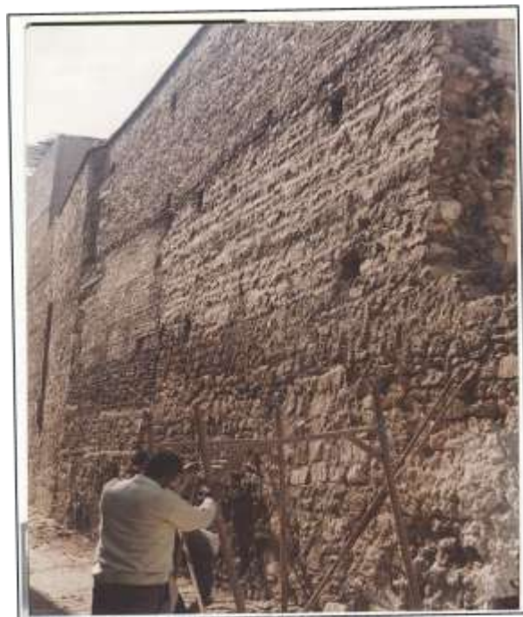
Figure (11). Present state of Sultan El-Ghuri palace wall remains, before restoration processes.
