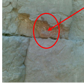
Fig. (7) Stress on the lower parts of Luxor temple's walls
