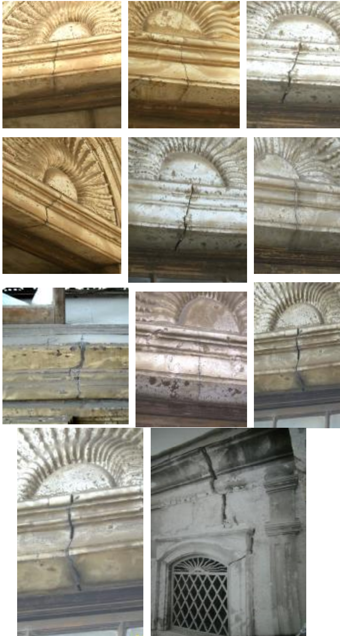
Figs. 32 - 42 Display cracks of 2 nd type in the springings of all lintels above openings in the mosque at positions of heavy load, the lower left photo. From Supreme Council of Antiquities archives (1935) .
