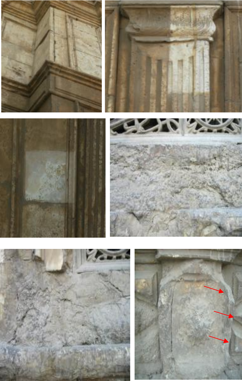
Figs. 102-107 Muhammad Ali Mosque show that the soiling areas easily removed and another type of soiling is not easily removed , also here there is a thick black crusts of irregular shape or discoloration (soiling) to crust are just an extreme case of the lower right photo , Since such crusts are brittle and tend to detach from the alabaster (red arrows) .
