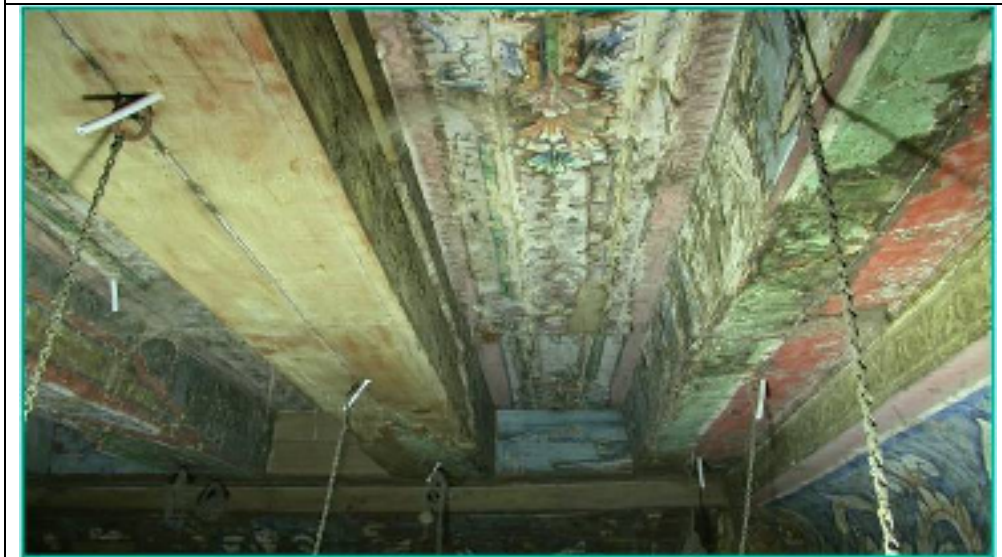
Fig. 7 A- D Shows the QC, decoration of Al Ashraf- Bersbay Madrasa, “notice the severe deterioration “.
