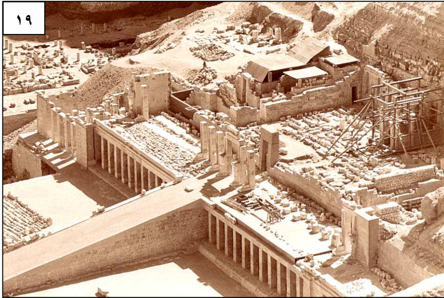
Fig. 19 Temple of Hatshepsut(Upper Terrace) at the beginning of works on the temple in (PCMA Archives)
